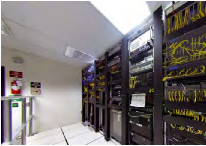
Telecommunication and computer areas
